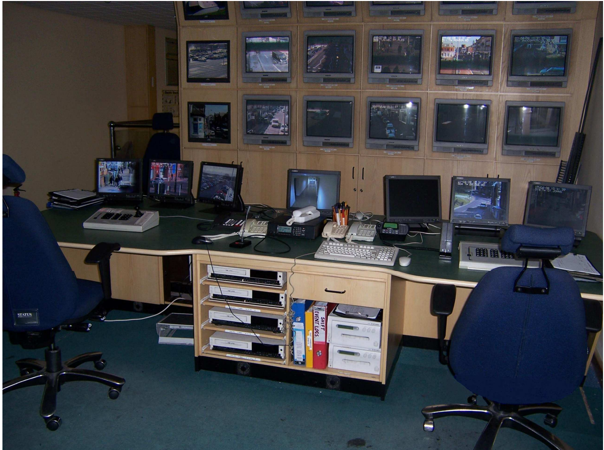
CCTV Control Room
